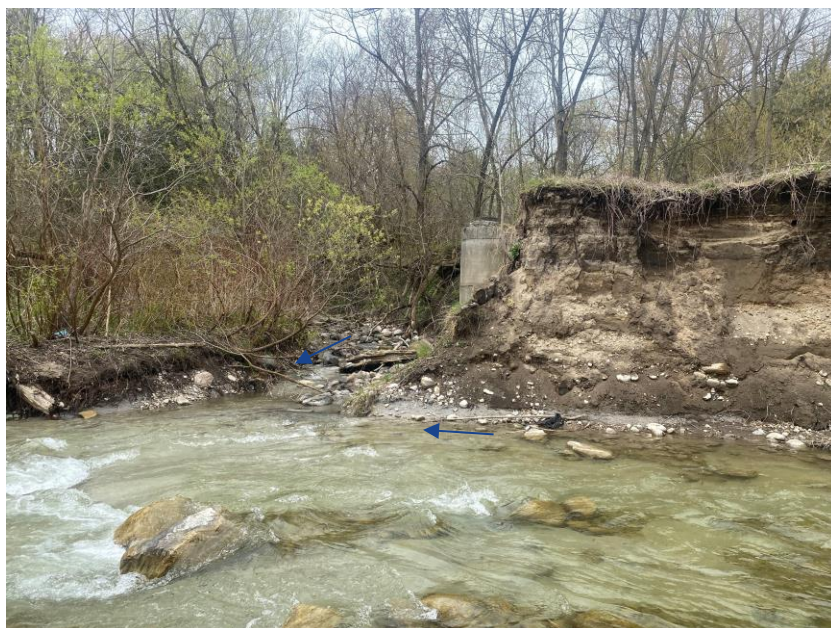
Photo 3. Looking westward towards the confluence of Bowmanville Creek (foreground) and Brookhill Tributary (background). The high outer bank of Bowmanville Creek, composed mainly of erodible pond-deposited sands, is near-vertical and is not easily overtopped by flood flows. Bowmanville Creek is migrating towards the manhole chimney.
