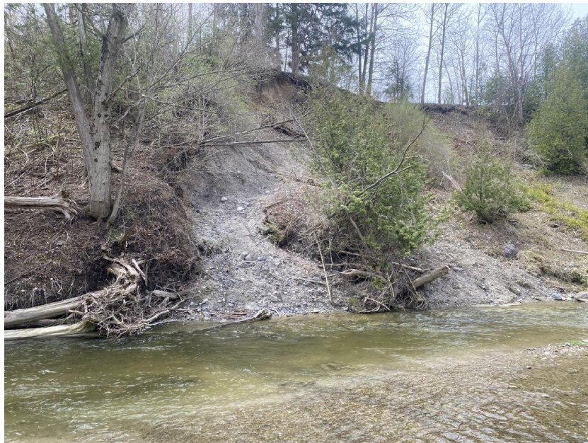
Photo 1. A slope failure near the northwestern property limit. The material deposited near the toe of slope is predominantly colluviated till.
