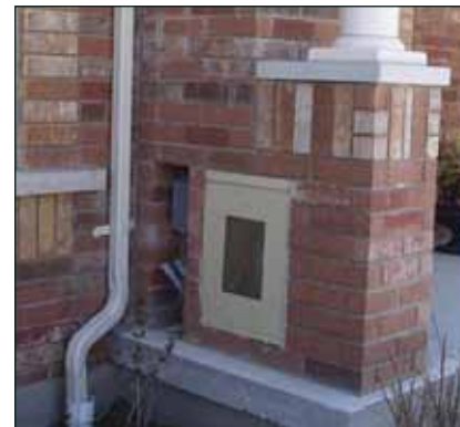
EXAMPLE OF RECESSED GAS METER
