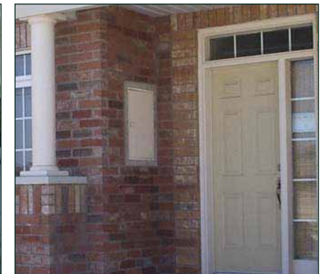
EXAMPLE OF RECESSED HYDRO METER
