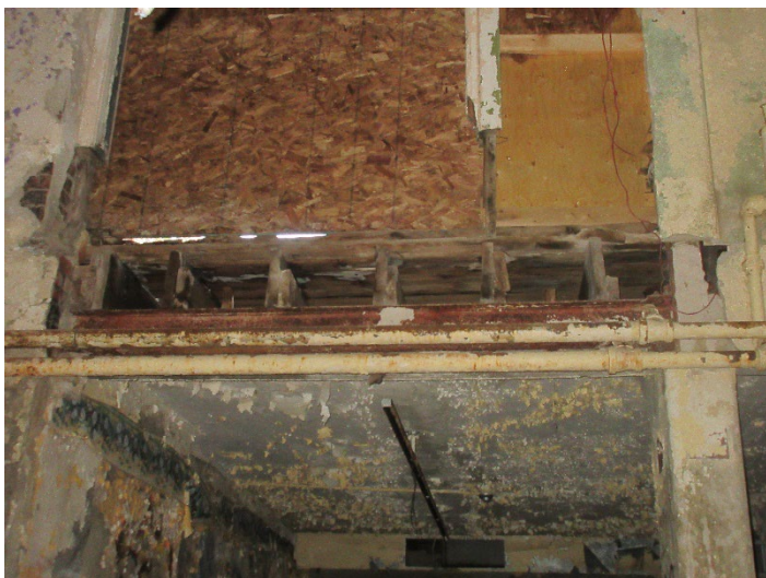
Photo 005 – Exposed Transfer Beam with Water Damage Visible
