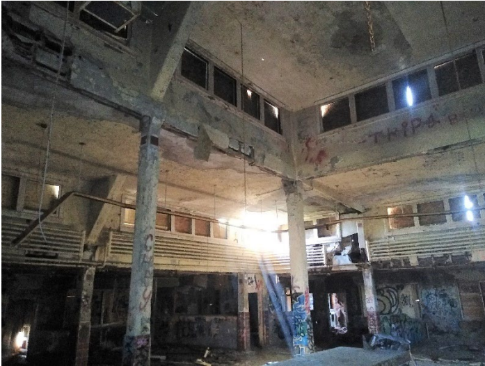
Photo 001 – Visible Water Staining Throughout Structure
