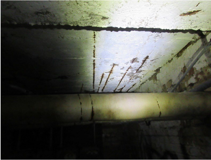
Photo 013 – Exposed Rebar on Underside of Suspended Slab
