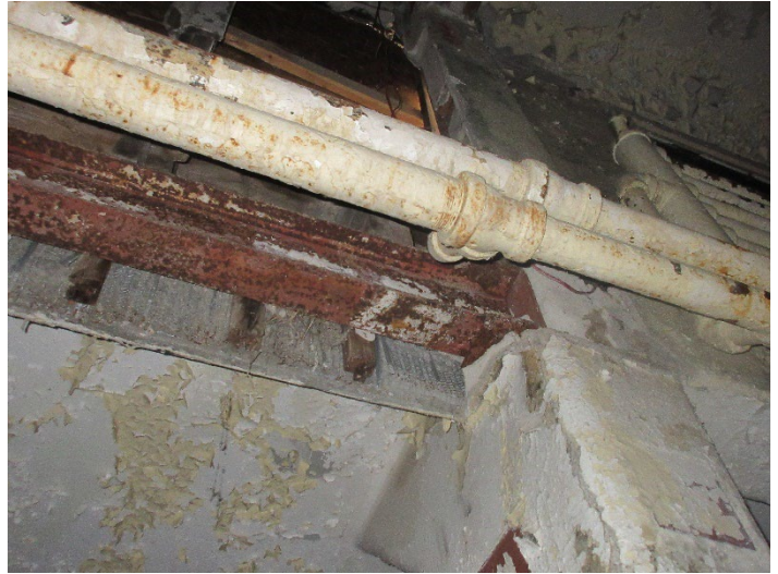
Photo 010 – Corrosion of Exposed Transfer Beam Supporting Clerestory
