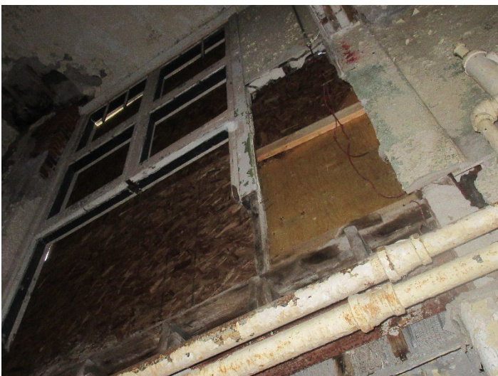
Photo 011 – Boarded Windows of Clerestory
