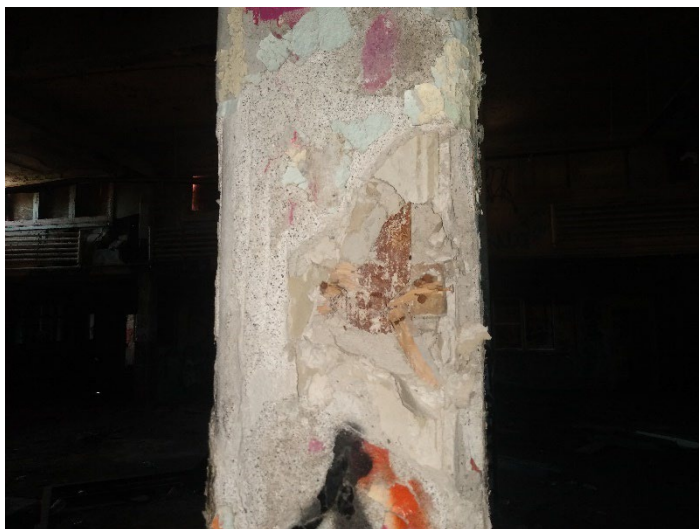
Photo 008 – Damage to Concrete Encasement
