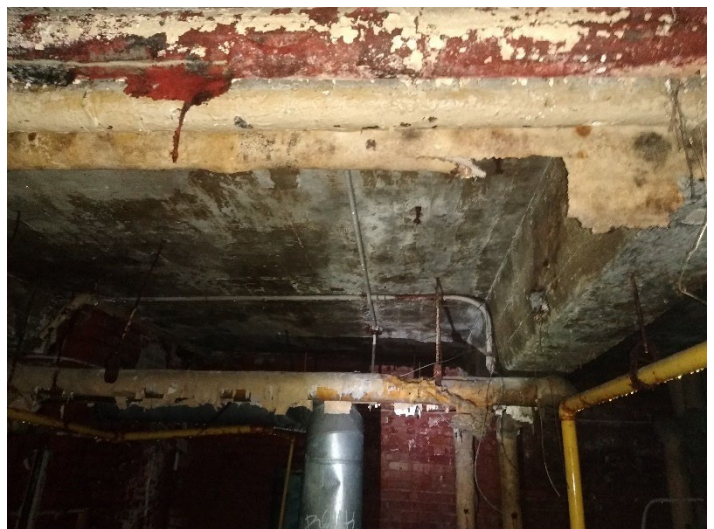
Photo 012 – Moisture Infiltration of Suspended Slab
