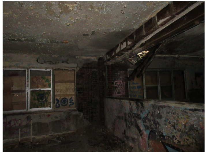
Photo 004 – Excessive Deterioration and Local Failure of Rafters (2/2)
