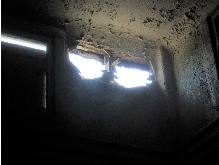
Photo 009 – Failure of Exterior Cladding
