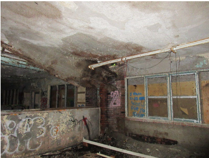
Photo 003 – Excessive Deterioration and Local Failure of Rafters (1/2)
