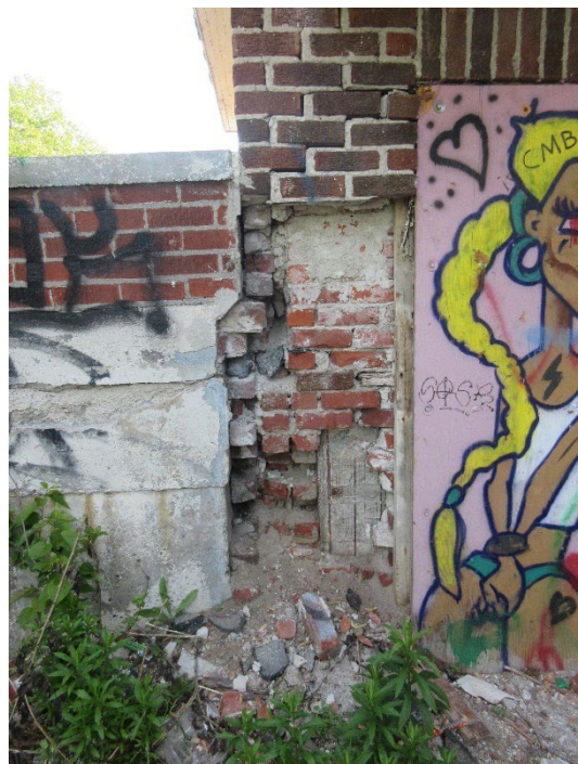
Photo 016 – External Brick Masonry Wall Damage (1/3)
