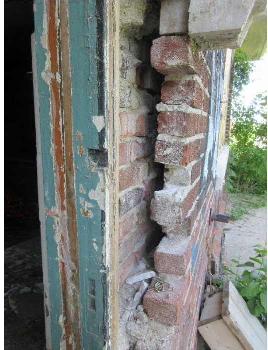
Photo 018 – External Brick Masonry Wall Damage (3/3)
