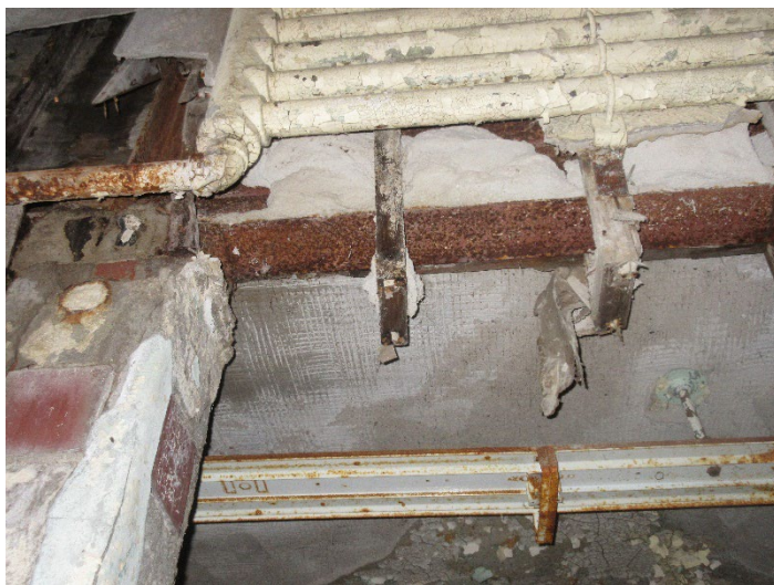
Photo 006 – Corrosion of Exposed Transfer Beam
