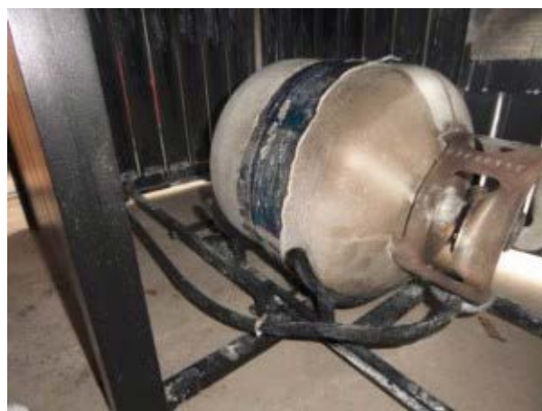
Propane cylinder and horizontal cradle assembly
