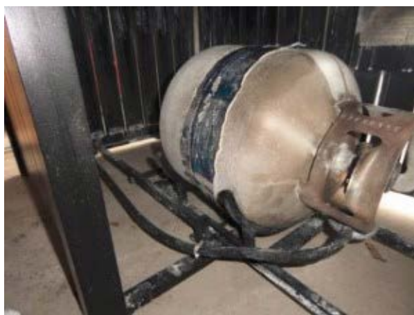
Propane cylinder and horizontal cradle assembly
